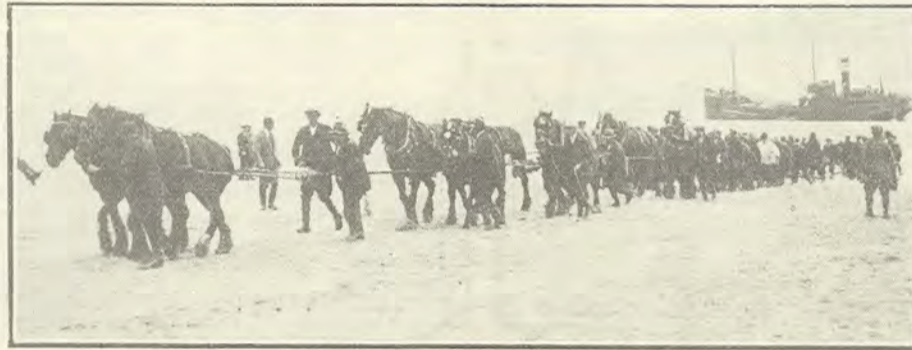
Hauling ashore the new Land's End to Newfoundland cable from the cable ship "Clyde Firth" (seen on right) at Sennen Cove, Cornwall.
